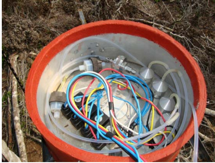
Figure 5 – Shelter Box installed in the top of the tower: manifold, electrovalves, filters, pre-filters for retention of particulate materials.
