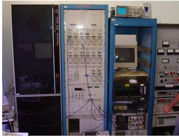
Figure 2. Fortaleza station control rack.
