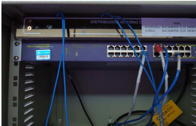
Figure 4. High speed network switch.
