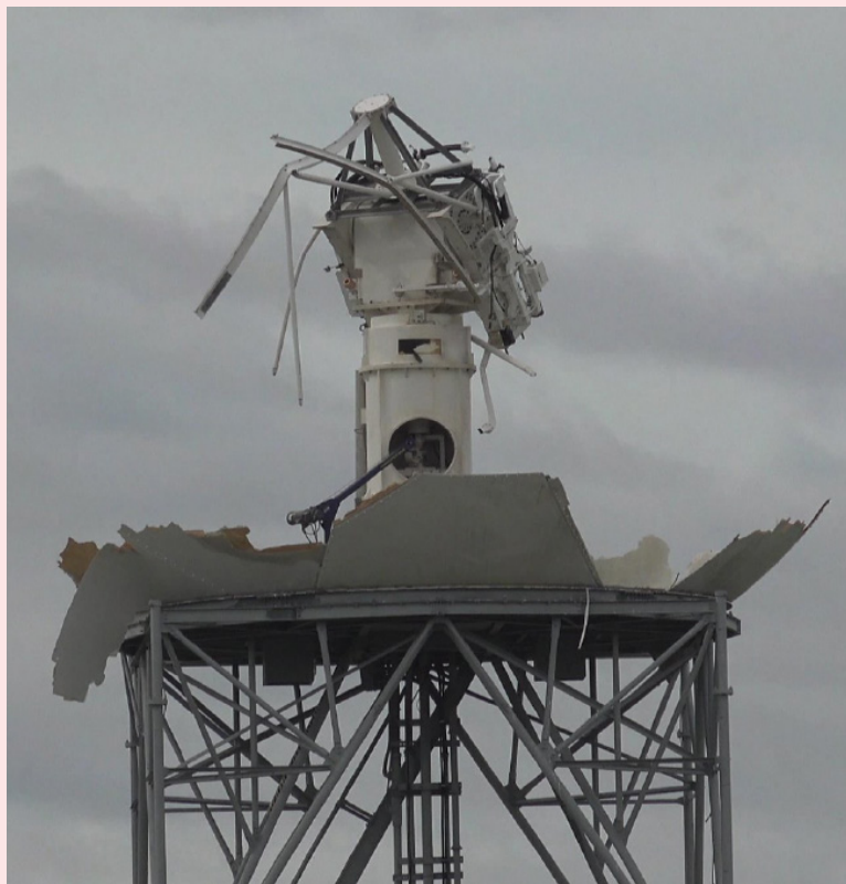
Fig. SB4.2. Heavily damaged National Weather Service Lake Charles radar following Hurricane Laura. (Image courtesy of Brett Adair, Live Storms Media.)
