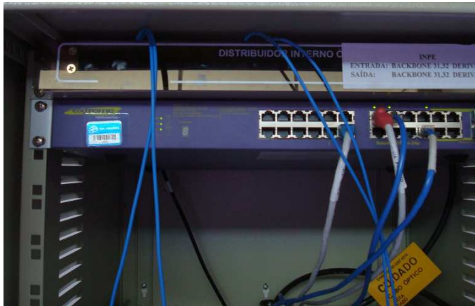
Figure 4. High speed network switch.
