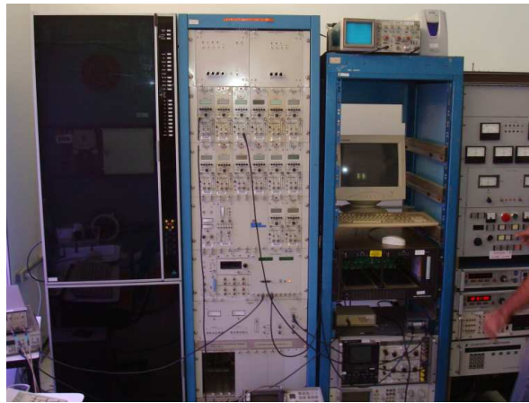
Figure 2. Fortaleza station control rack.
